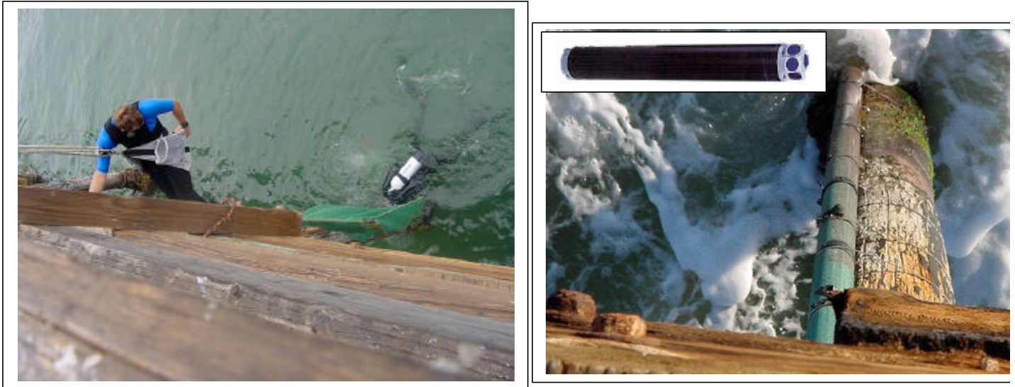
Figure 4. Left. Photograph of divers installing the equipment onto a piling on the south side of the Imperial Beach Pier (divers: Millikan and Terrill). Axel Pierson is suspended from a bosun's chair and is guiding the hardware into place. Right. What the current meter looks like when mounted to the pier piling. The current meter (see inset) fits into the end of a copper/nickel pipe with the sensing head sticking 2" out of the end. This pipe is banded to the wood piling by stainless steel bands. The instrument is protected from the elements inside the pipe and has already withstood the forces of several winter storms.
